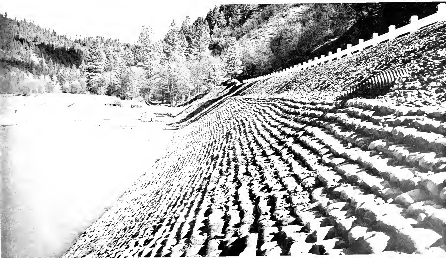
The above pictures show portions of 25 acres of sacked concrete slope paving placed on the banks of Trinity River for protection of the highway at flood stages. A total of 148,029 sacks was laid, approximately one sack per square foot
